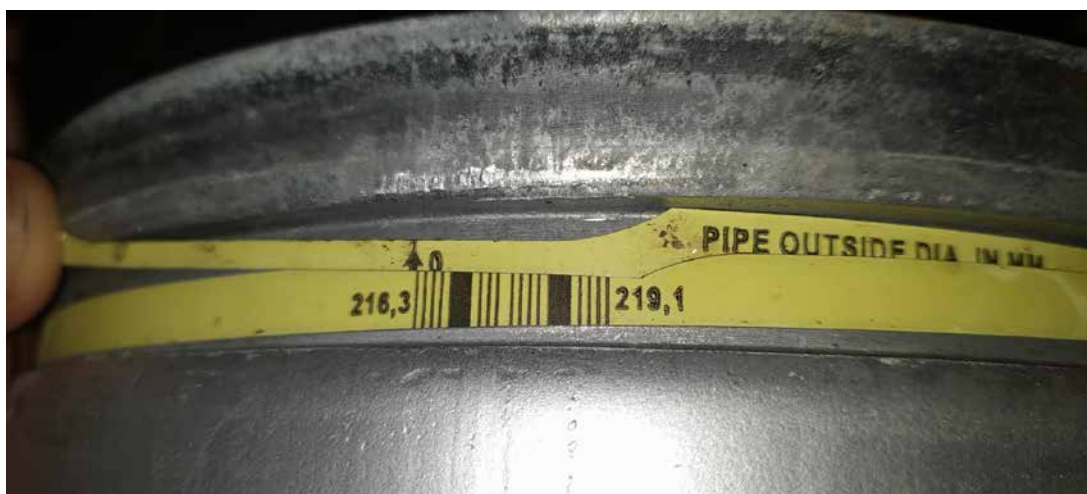
Example photo of over grooved pipe.
