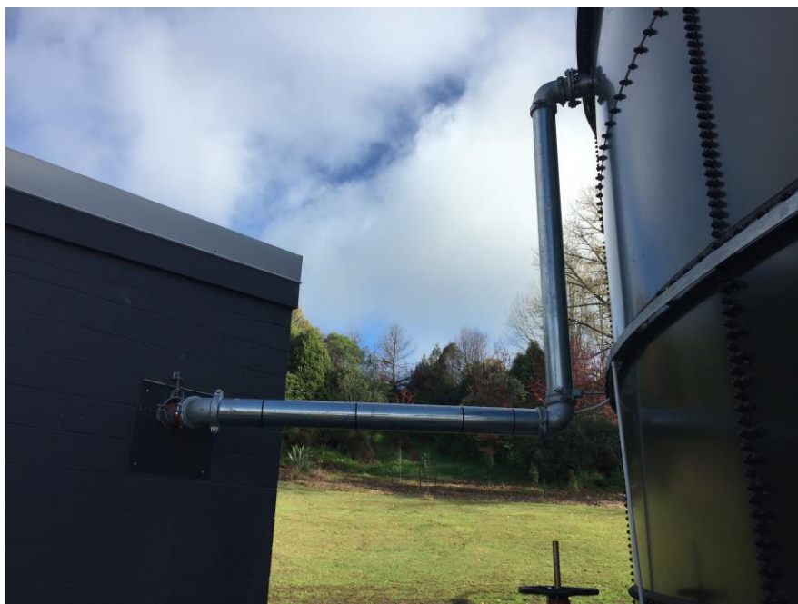
Figure 1 – Lack of independent support and bracing.
