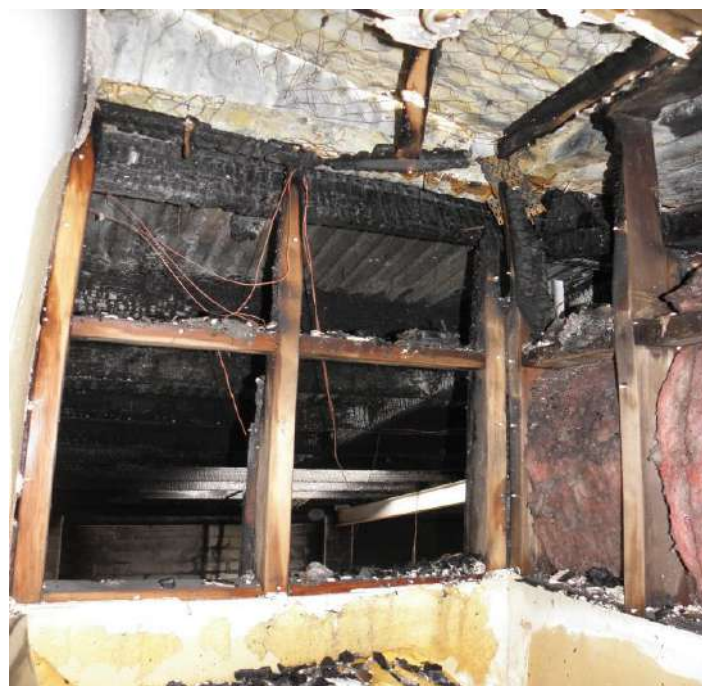
Figure 2 - First Incident: remnants of the wall separating the kitchen of the residential unit from the workshop
