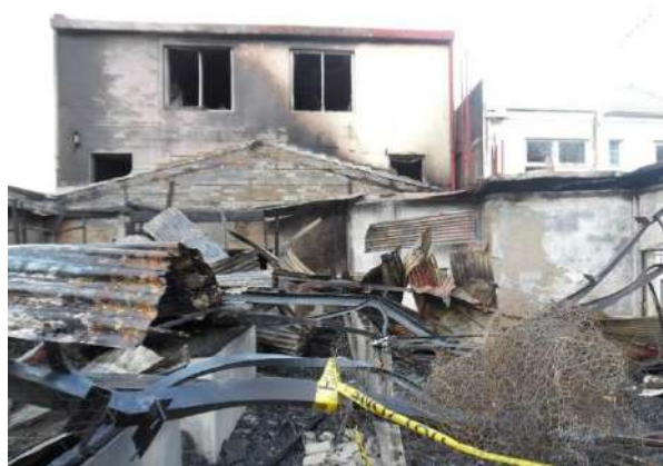
Figure 1 - Second Incident: Rear facade of commercial unit overlooking the burnt out workshop
