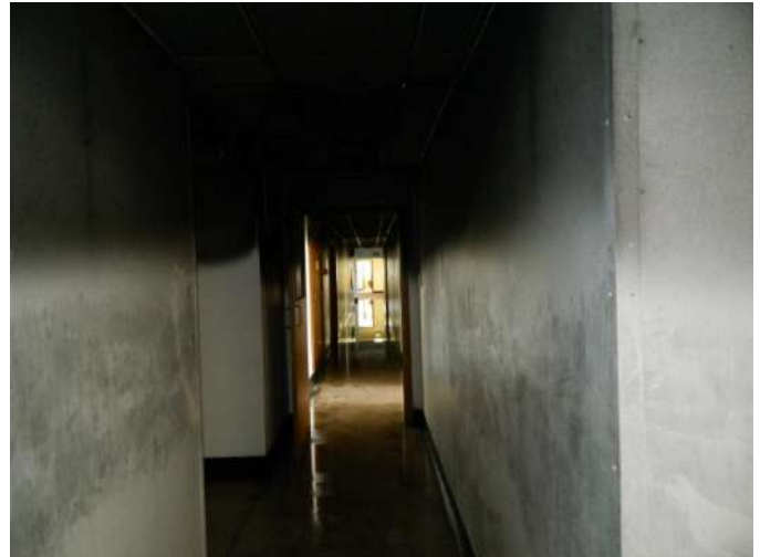
Figure 2: Showing extensive smoke damage throughout building
