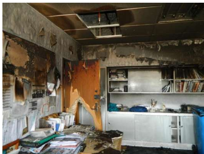
Figure 1: Room of origin of fire
