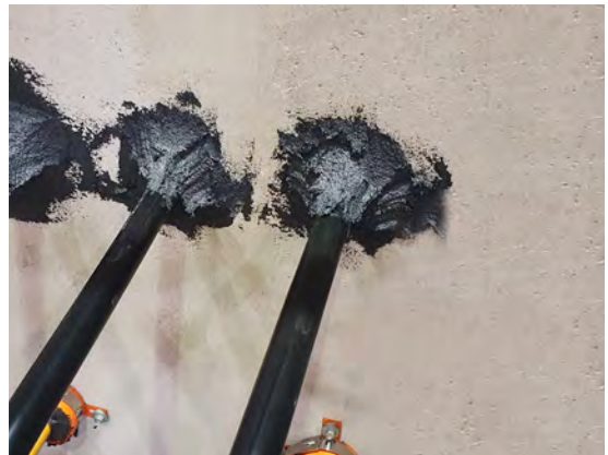
FyrePEX TM HP Sealant applied to depth of at least 60mm from one side of the wall with fillets if required.
