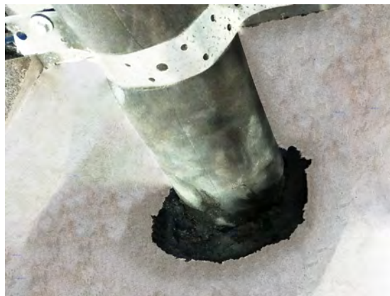
FyrePEX TM HP Sealant applied to depth of at least 60mm from top side of floor slab.
