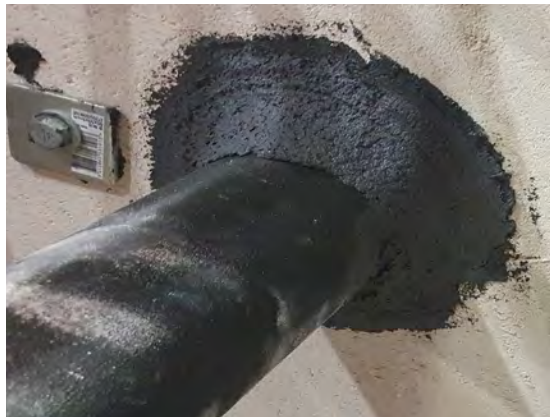
FyrePEX TM HP Sealant applied to depth of at least 60mm from one side of the wall with fillets if required.
