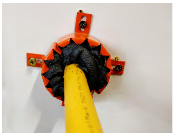
Metal sheath secured to plasterboard wall using minimum 8gx25mm screw fixings. FyrePEX™ HP Sealant to be filled into a metal sheath from each side of the wall. Refer to service specific requirements on pages 5 and 6 .
