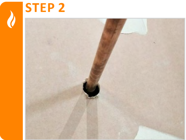
Run services through the holes formed, ensure the pipes are nominally centered in the opening. Clean the penetration of dust.
