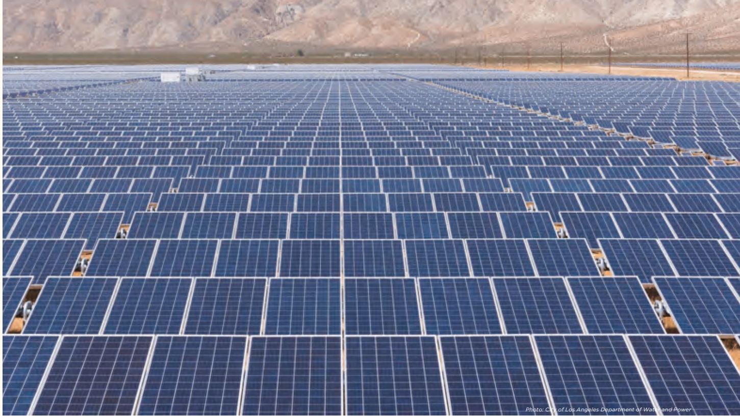
Photo: City of Los Angeles Department of Water and Power
